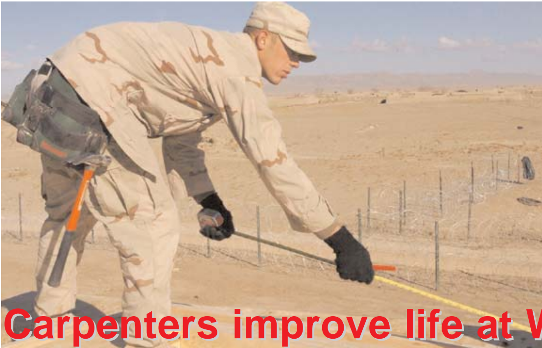
Left - Spc. David Baker, a carpenter from the 367th Eng. Bn., uses a tape measure to check the dimensions on a new guard tower at Waza Khwa, Afghanistan.
